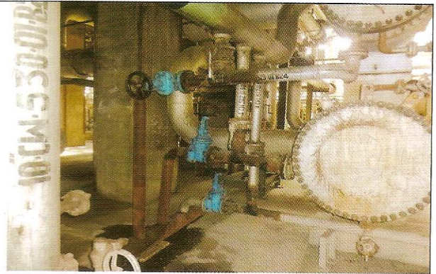
Figure 8 – Back flushing arrangement in E-3405
