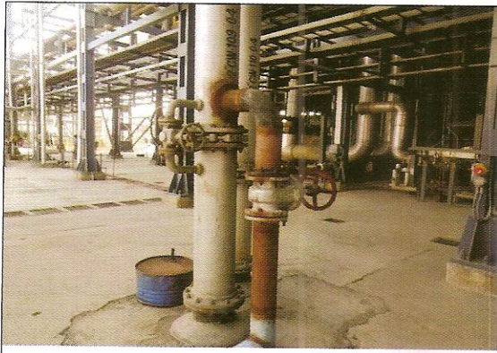
Figure 7 – Back flushing arrangement in -E-3312
