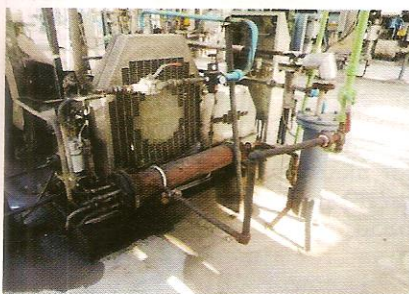
Figure 12 – Water cooled inter stage coolers
